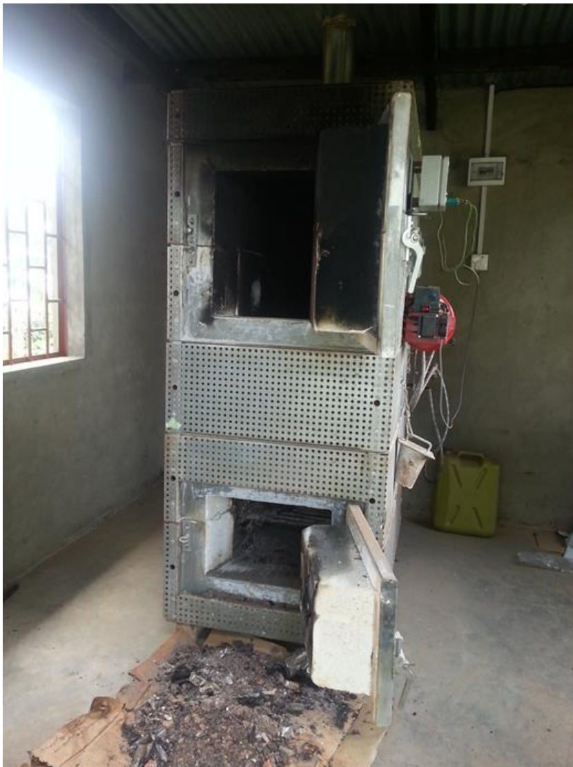
Photo 4.8: Incinerator installed at the hospital behind the TB ward
