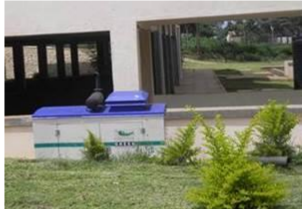
Photo 4.2: One of the standby generators located near the proposed project site
